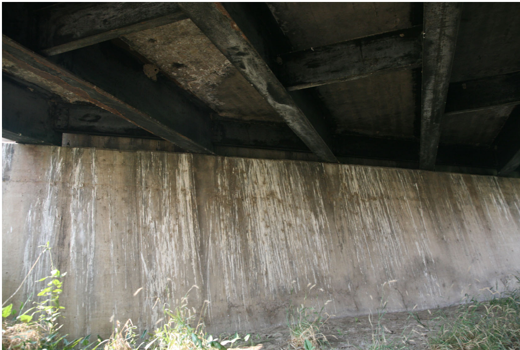
Picture 3 – Corrosion, cracking, efflorescence
